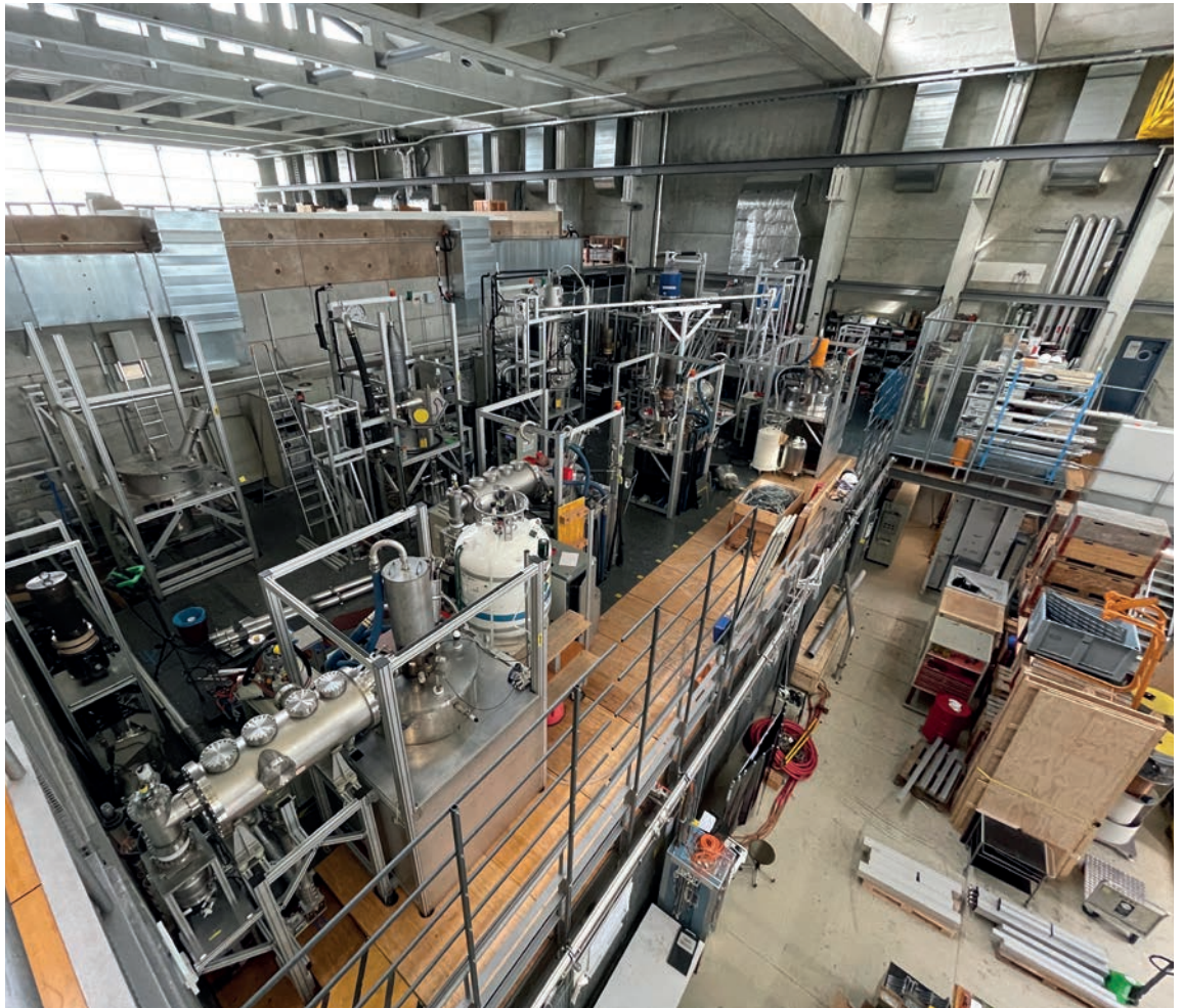
2 Overview of the gyrotron platform, taken during the installation of the neutron radiation shield. The TCV tokamak hall is beyond the wall to the left.
